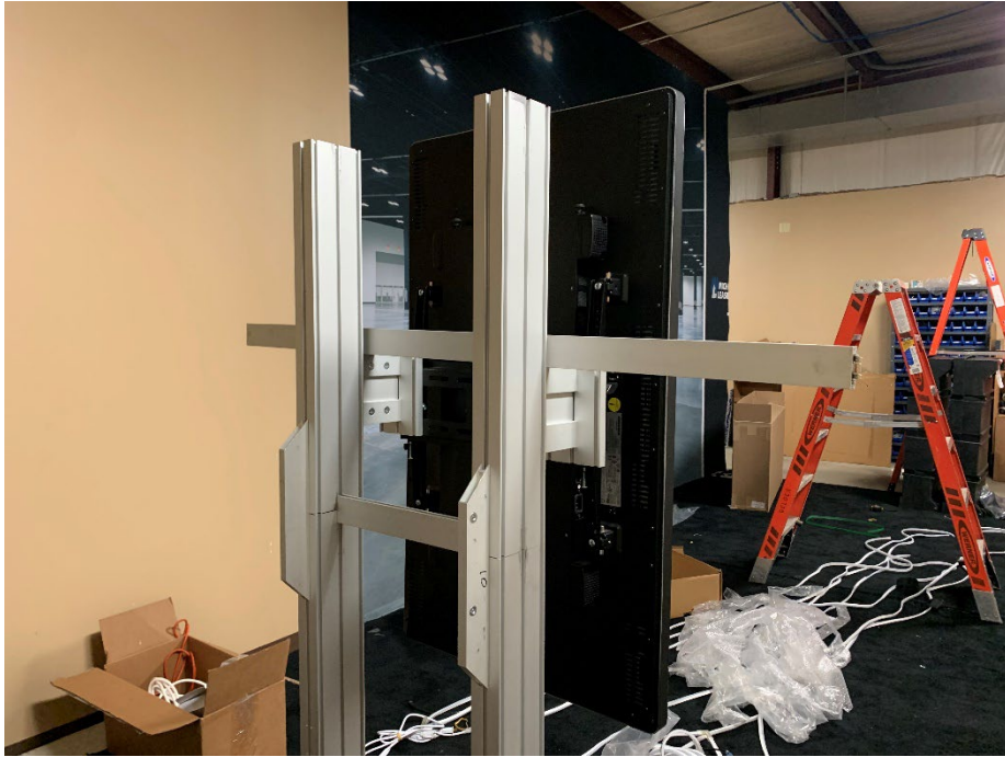
(1) Pch1174mm (B3) connect to frame that houses graphics. This will be internal, sandwiched between graphics (see photo below).
